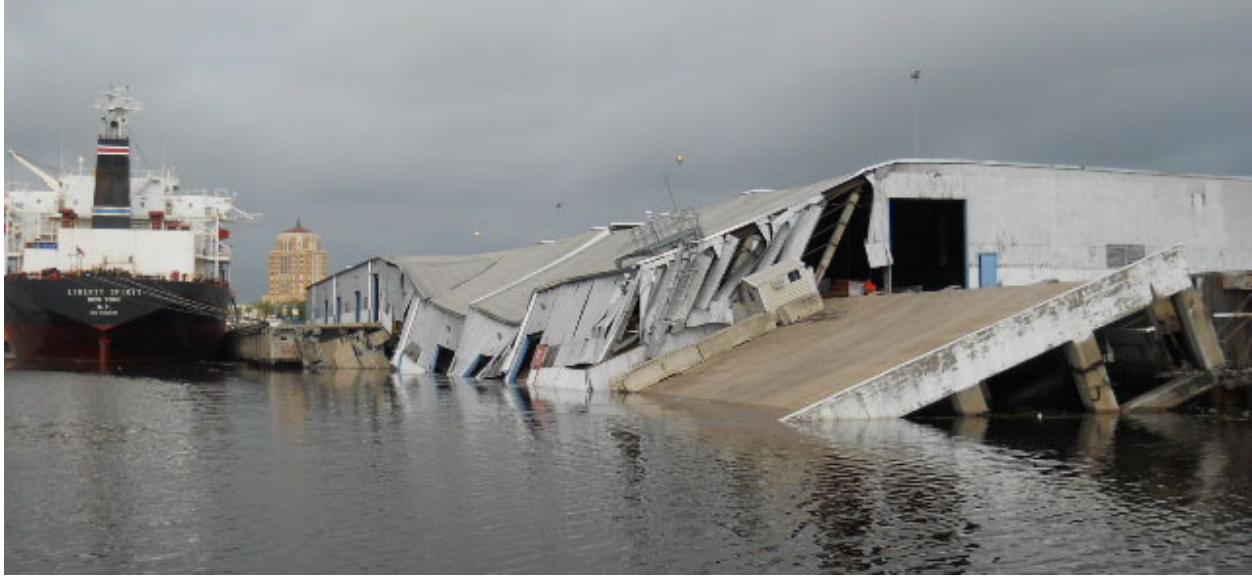
Figure 4: POB – Collapsed Dock 4 Structure & Shed – March 2012
