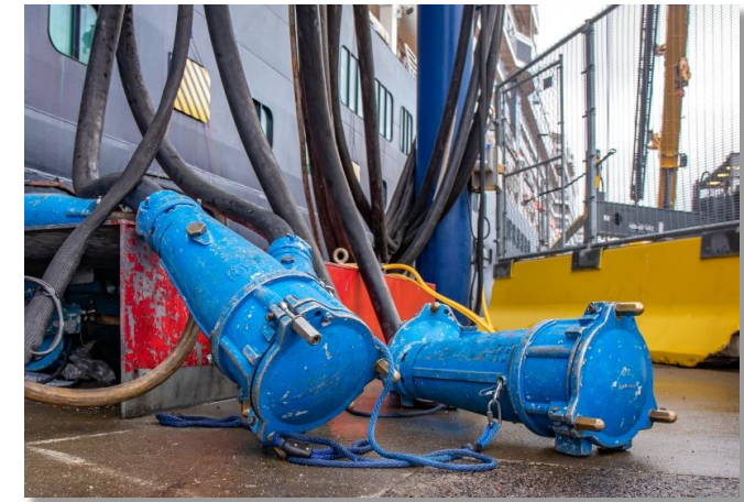
Shore power at the Port of Seattle
